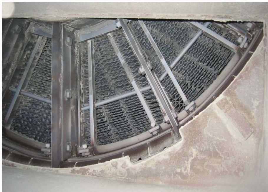
Figure 5a: Pilot Air Preheater Cold-End Basket Flue Gas Exit with Mg(OH) 2 Injection
