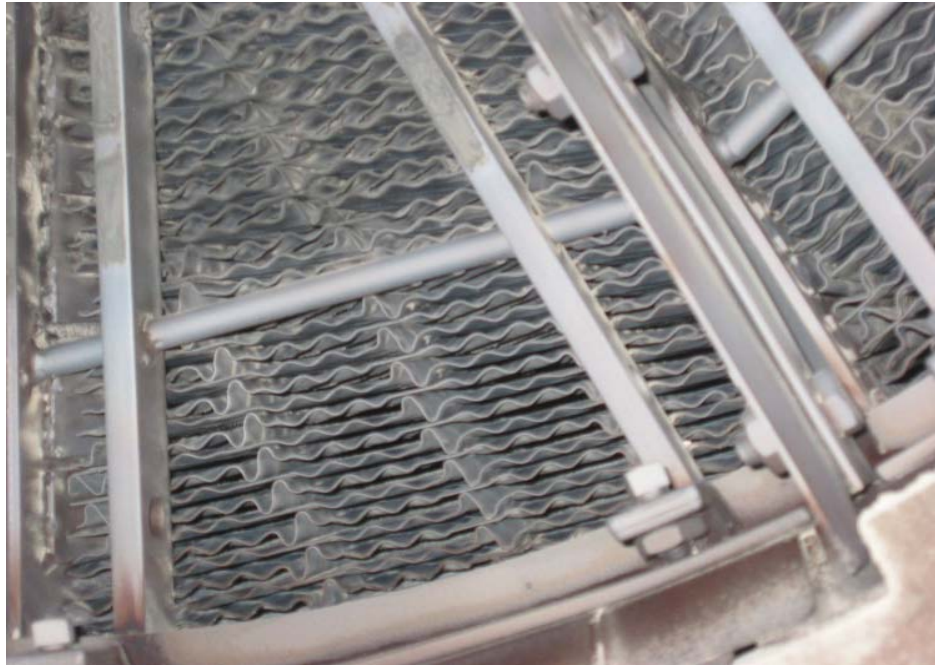
Figure 5b: Pilot Air Preheater Cold-End Basket Flue Gas Exit with Mg(OH)_2 Injection
