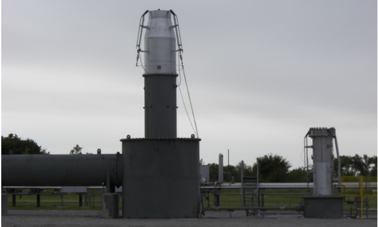
Figure 4-3. Flare Burners. Air-assisted on left and steam-assisted on right
