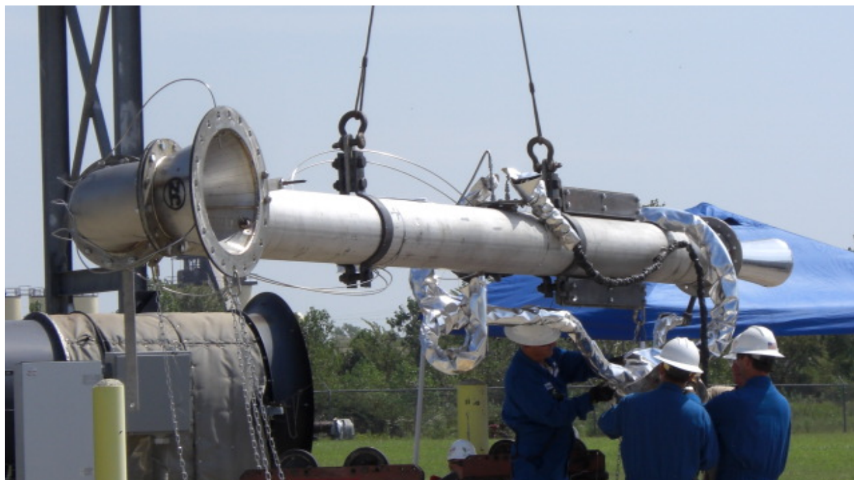
Figure 4-8. Sample Collector at Near Ground Level. Collector inlet is at foreground and eductor is at far end. In photo, Zink personnel make adjustments to heated transfer line supports. Shackles and cable at center allow crane to lift and position Sample Collector.
