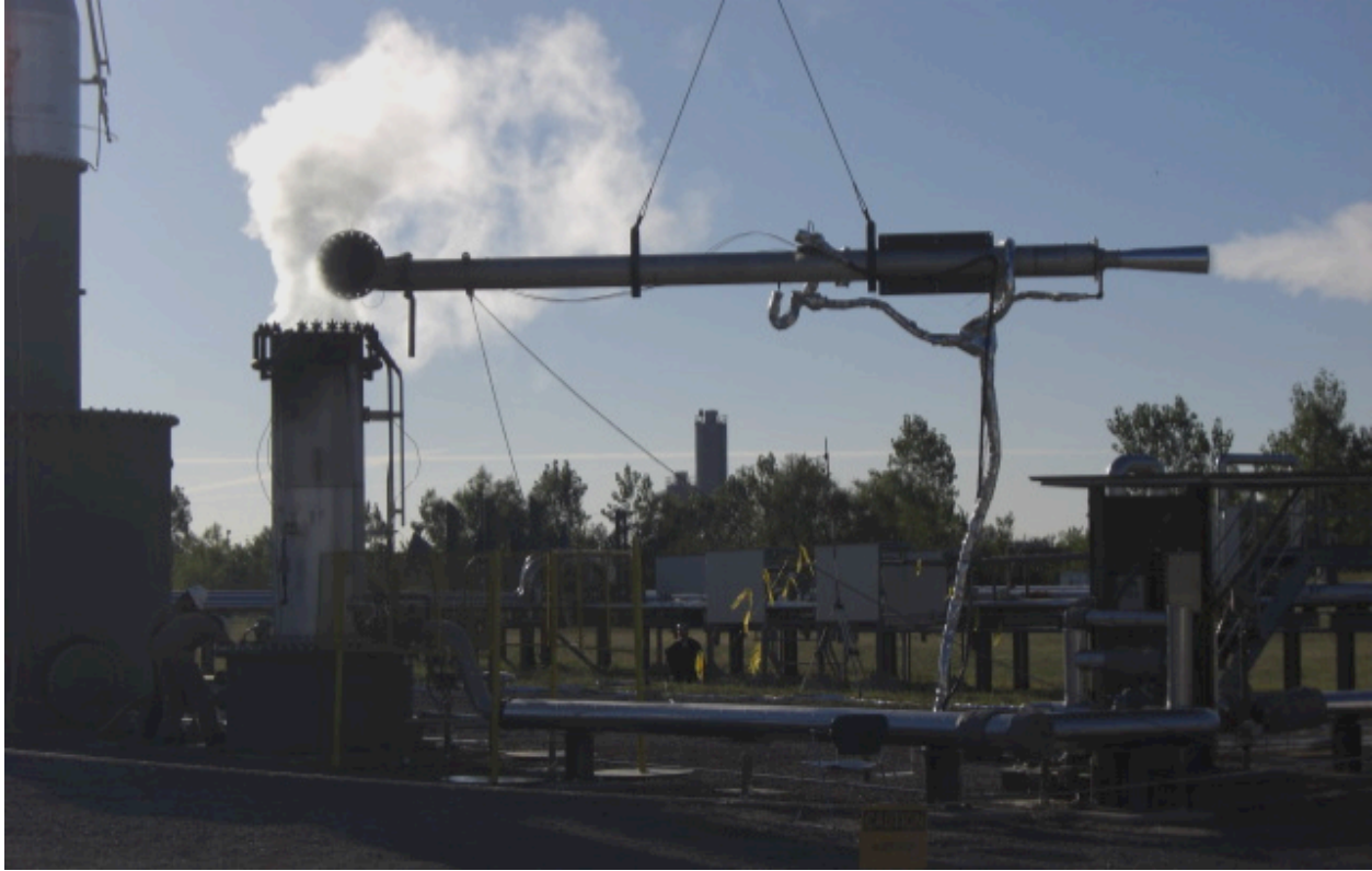
Figure 4-2. Flare Plume Sampling System During Morning Steam Only Start-up Routine
